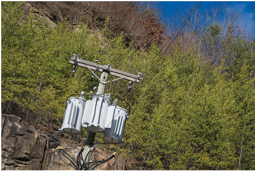
Transformers belonging to AEP's Kentucky Power Company were photographed near the old Ermine Grade School in Whitesburg Monday. (Photo by Malcolm J. Wilson)
