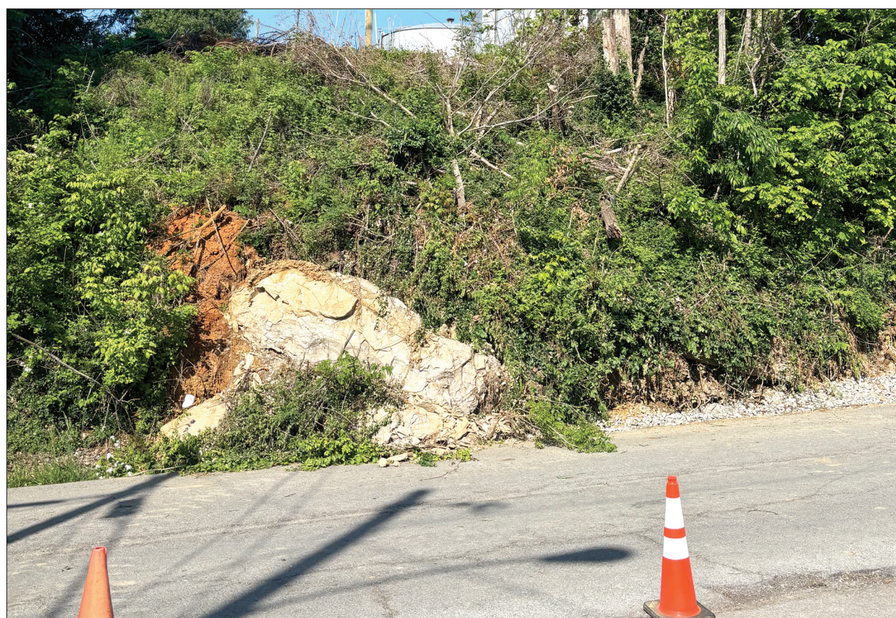
West Hodgenville Avenue from Second Street to Hidden Valley Road is closed. The small hillside near the water tower has fallen very near to the edge of the road making any traffic a potentially dangerous situation. Residents of Graham Court and Lewis Court, two of the nearby neighborhoods, have been forced to use the lower entrance to their homes and cannot access their homes coming from the area near Adanta and the Cumberland Presbyterian Church.
