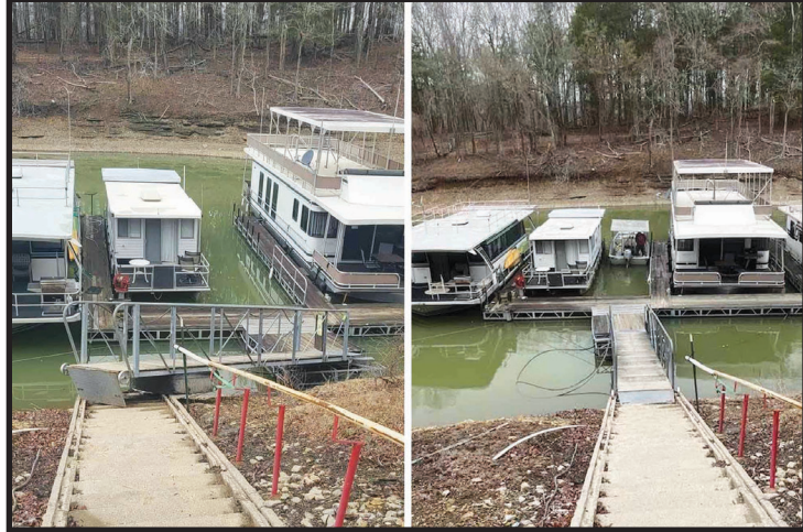
Before and after: The team of Kingfisher Marine recently fixed the broken anchor of the dock at Holmes Bend Marina. (Photo source: Kingfisher Marine)
